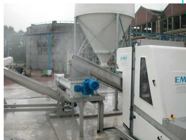
Chaulage / Compostage Liming / Composting
