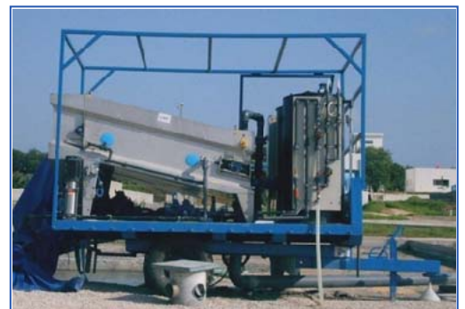
Mobile sludge thickening station before drying beds
