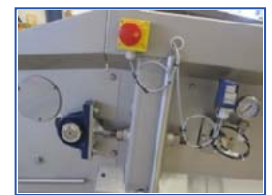
Belt tensioning and washing systems
